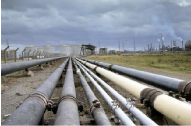
Oil pipes, Seal Sands, c.1995.
