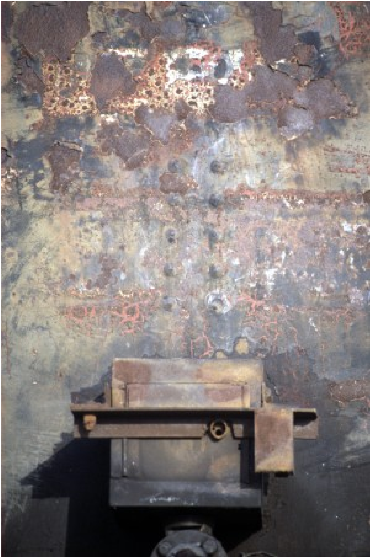
Rusting surfaces of a steel oil tank and a corrugated iron shed. 1998.
