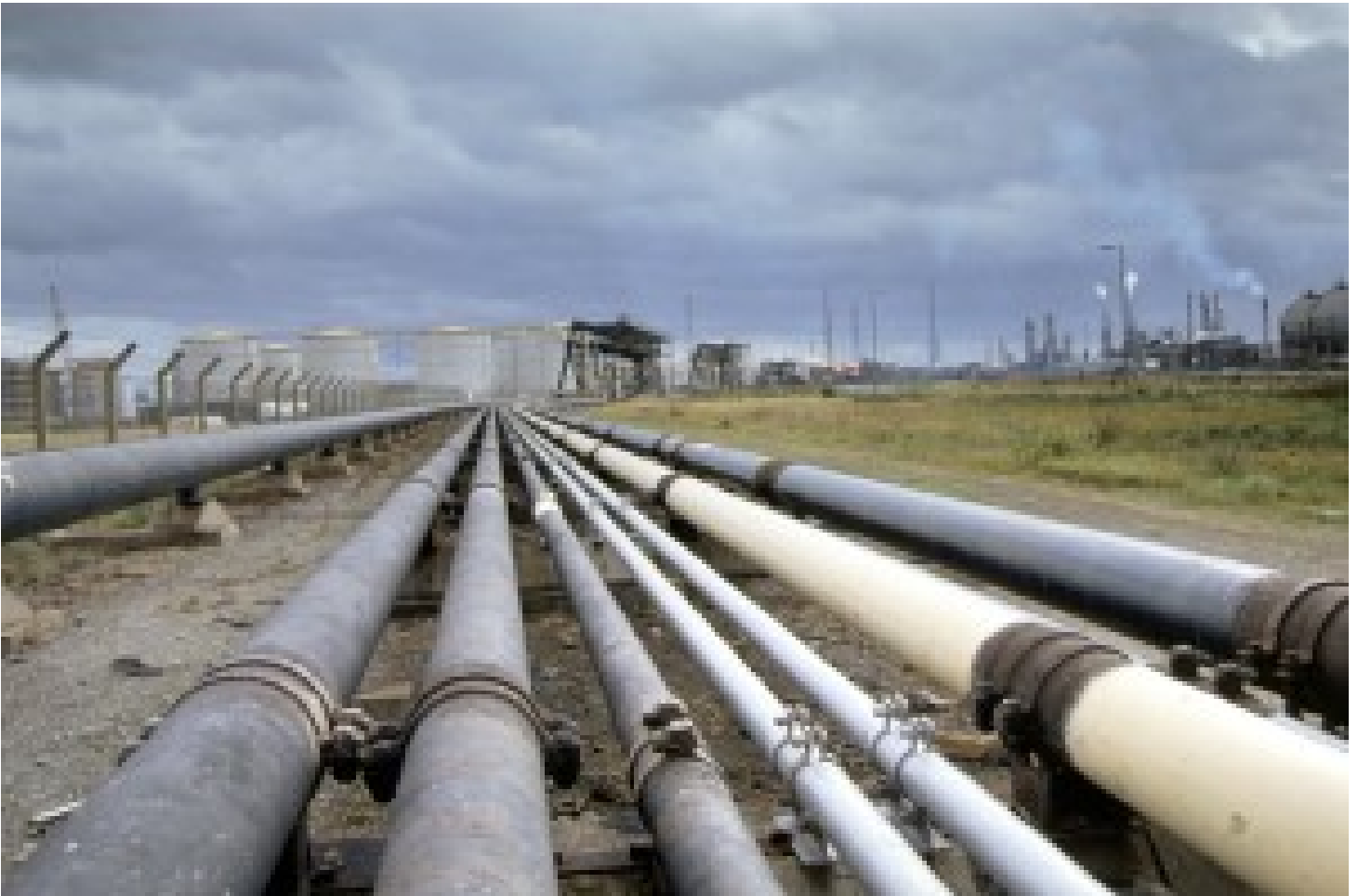
Oil pipes, Seal Sands, c.1995.
